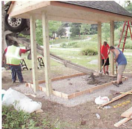
Ben Stewart (in the red shirt) and his dad Doug lay concrete in the new Baggage Cart Display Area.
