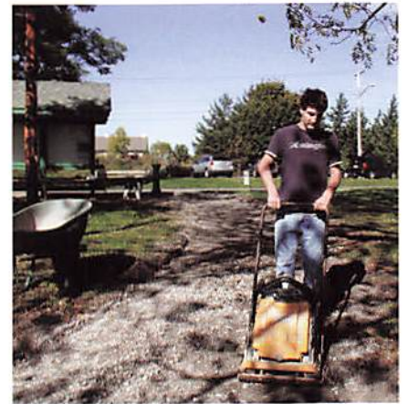
Colin Prato uses a plate compactor to settle the new pathway's stone base.
