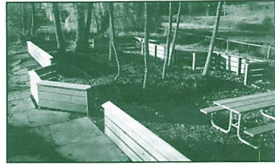
The knee wall at Rochester Junction built by Garrett Koek and 42 others required 337 man hours to construct.
