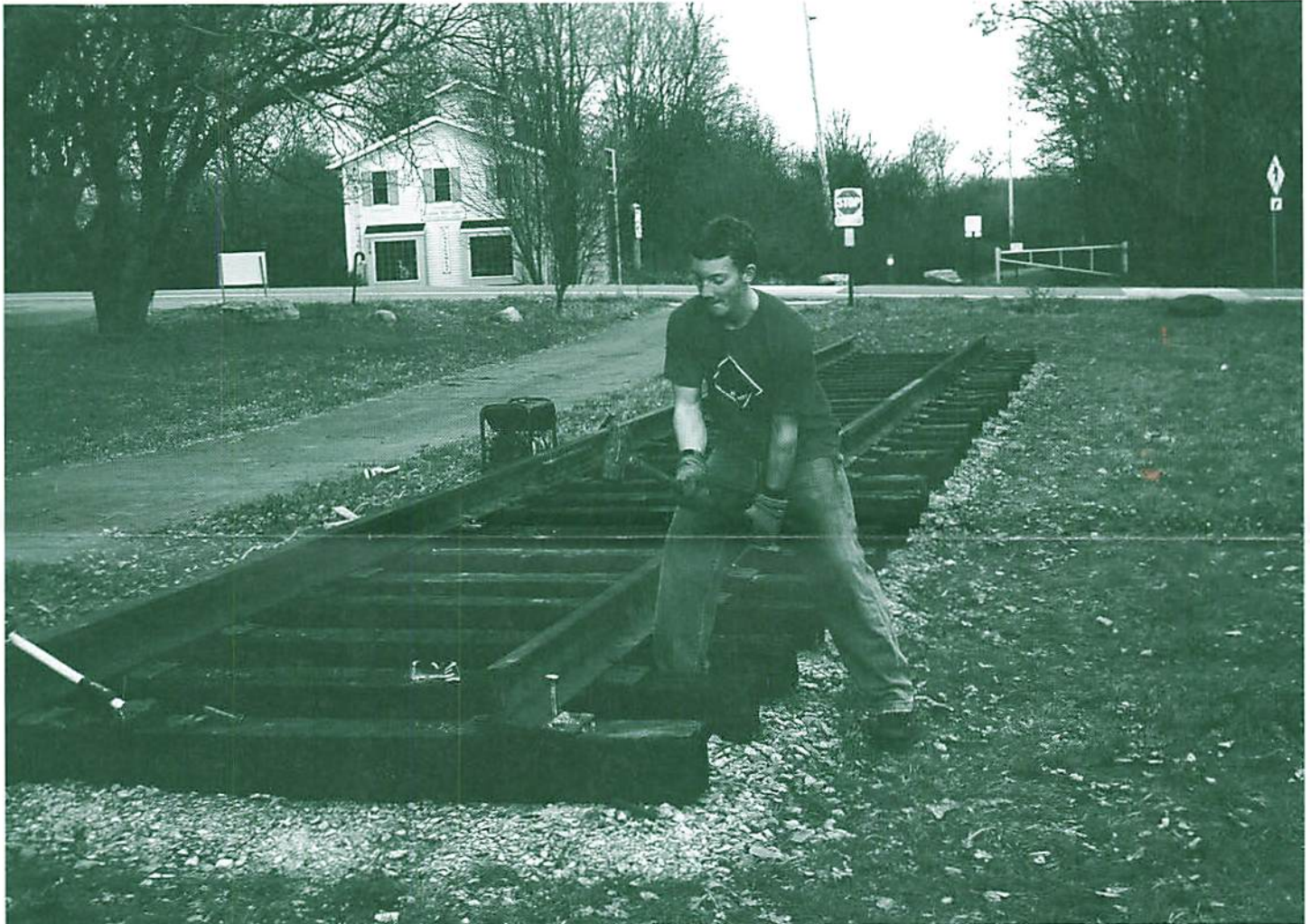
Sub-base, base, ties, and rails are all in place as Evan Schmidt drives the final spike in Mendon Station Park
