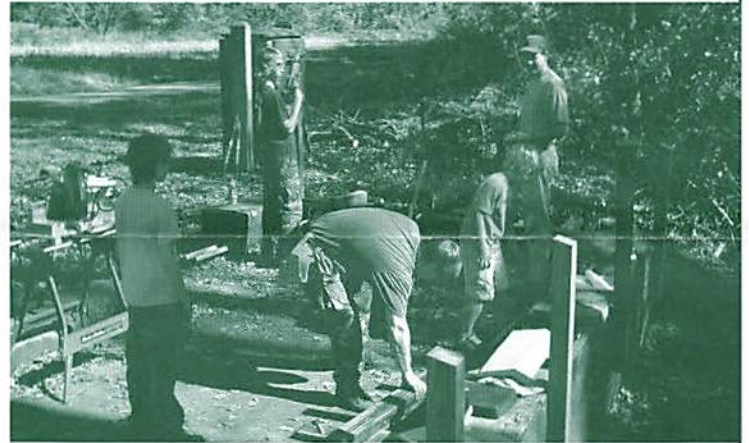
After digging out the old foundation, Scouts start construction of the knee-wall that will outline it.
