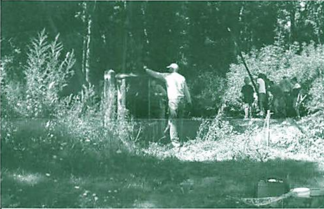
Interlocking Tower & Electrical Box (Completed) Eagle candidate Ethan Gardner and helpers start removing brush and debris from the foundation of the original tower.
