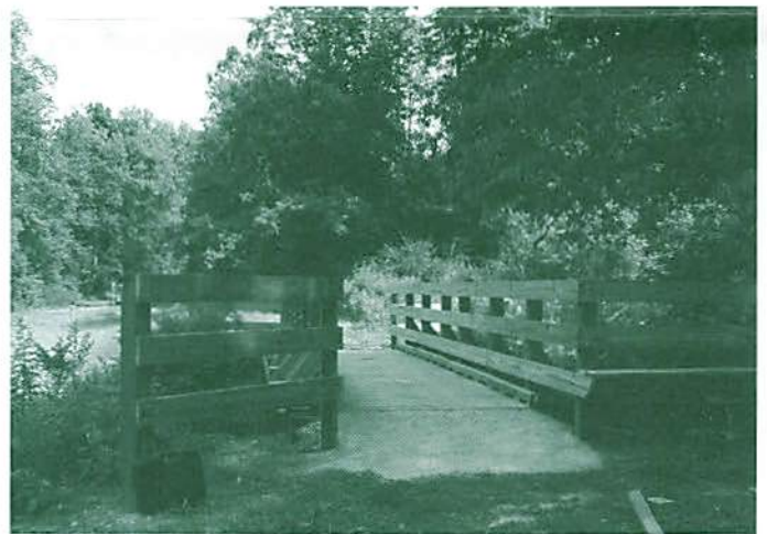
Sub-base, base, and ties all leveled and ready for rails to be attached.
