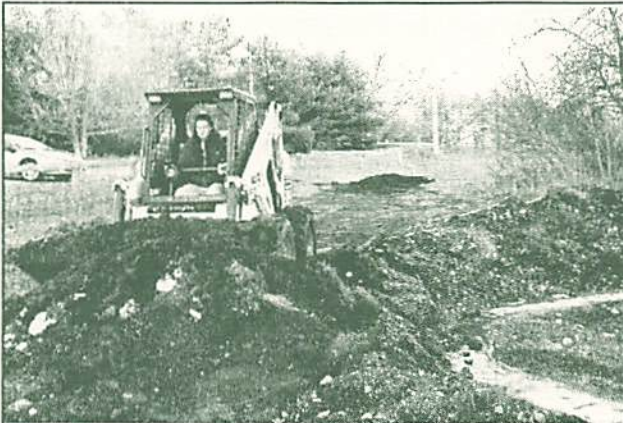
Darcy Gregg from Bears Outdoor Play Products donated her time and Bobcat to help with the first pavilion.
