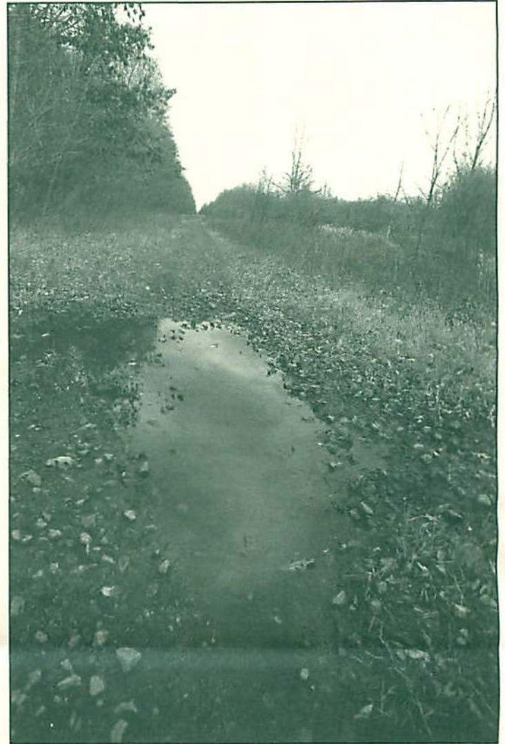
One area of the Trail flooded due to poor drainage
